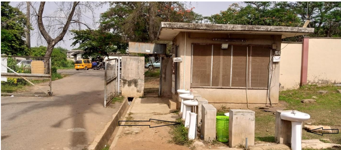
Dilapidating hand washing facility put in place during the COVID-19 period
